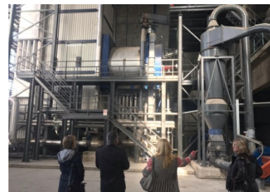
Figure 6. Biomass boiler room 18MW in TETO
